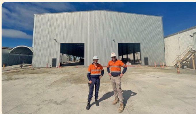
The new storage shed at the Port Lincoln Primary Distribution Centre (PDC) under construction.
