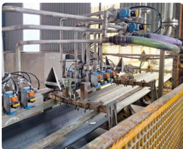
Liquid application line, Circular Head Distribution Centre.
